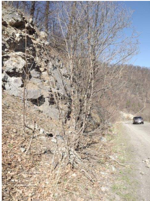
Fig. 10. Rockfall outside of village Vahagni
